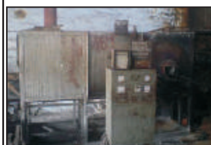
Fuel oil fired end bar reheating furnace
