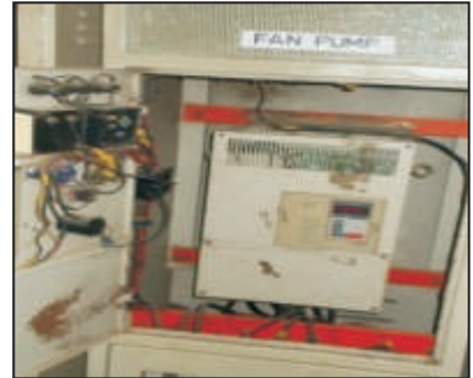
VFD Control Panel on Fan Pump 100 HP
