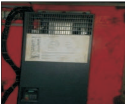
VFD Control Panel on 120 HP Energy Efficient motor
