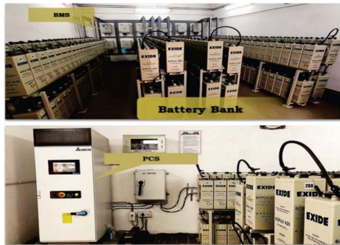
Figure 8- Battery Bank & Power Conversion System
