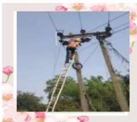
Disconnection Activities at RWSS point in TED Division
